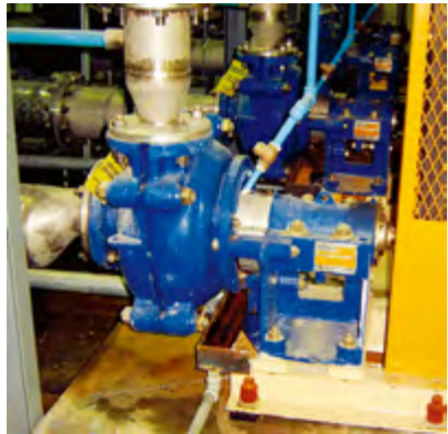
SH/50C slurry pump handling hot caustic slurry in an alumina plant.
