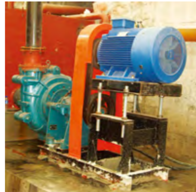
SH/150E slurry pump delivering fine coal to dewatering screen in a coal washery.
